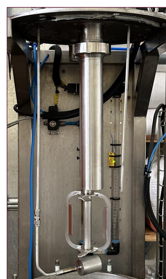
Figure 2: Sparger in digester.
